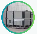
Genset with ATS Device
