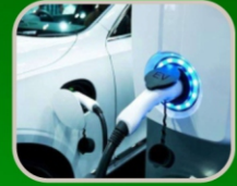
ELECTRIC VEHICLE CHARGING POINT
